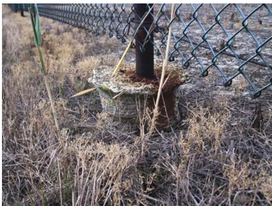
Photo 1. Fence post jacked up from ground near Sarnia area (SW Ontario)
